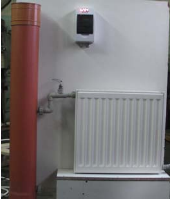
In-line water heater with a power of 3 kW
