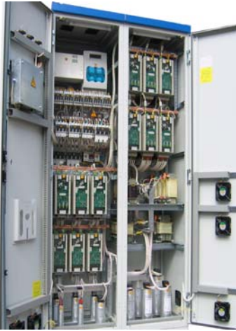
Control cabinet with ASDPFC
