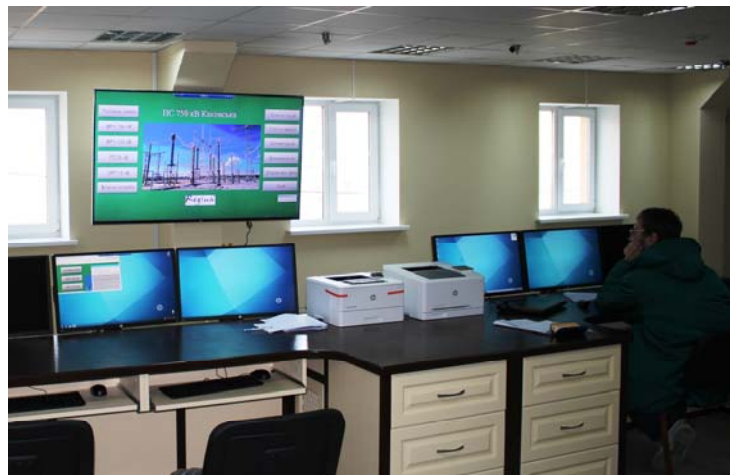
Control room of 750kV "Kakhovska" substation
